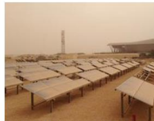
Figure 1 Dust accumulation on photovoltaic (PV) modules
